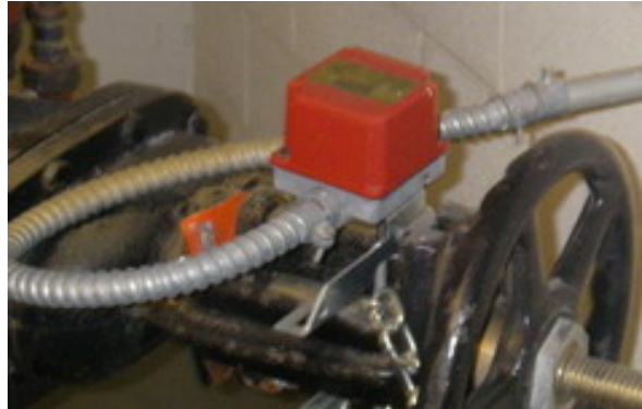
Tamper switch on a sprinkler valve
